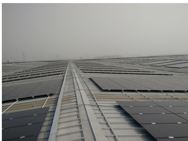
Zhejiang Jindun Fire Control Equipment Co. Ltd. Kapacitet: 4,0 MW Plats: Shaoxing, Zhejiang
